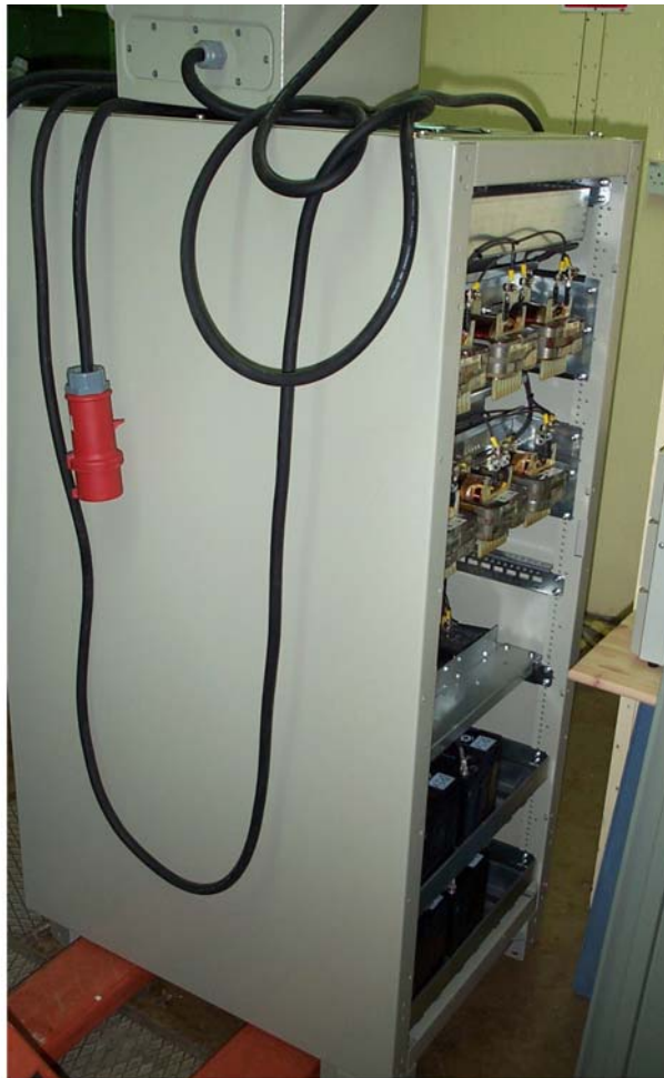
Right: rack with UPS system with removed front cover.
