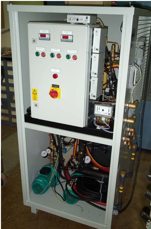
Fig. 8 Left: rack with coolunit, heat exchangers and waterpumps with removed front cover.
